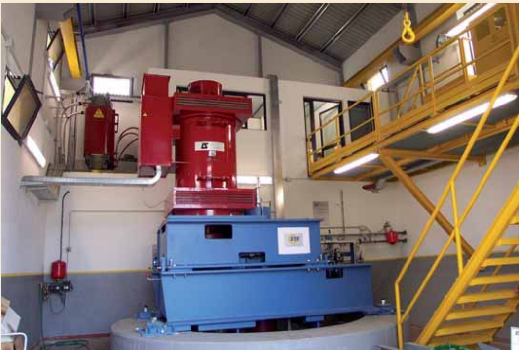
Figure 1: Inside hydropower view with a close-up of the alternator.
